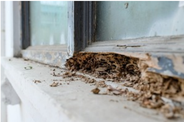
Termite damage on a wooden window frame. Attapon Thana/Shutterstock
